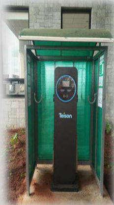
Electric Vehicle charging station
