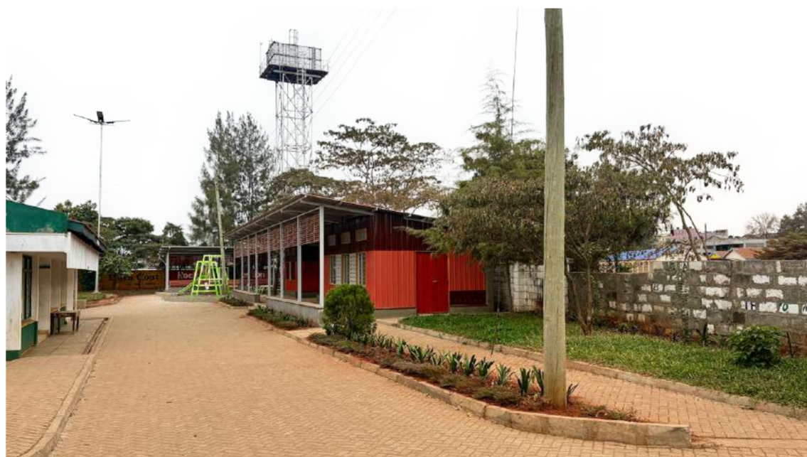
Kongo - Solar high mast lighting
